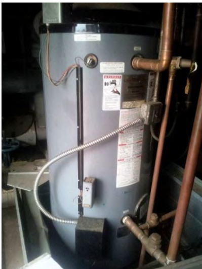
NEW HOT WATER HEATER
